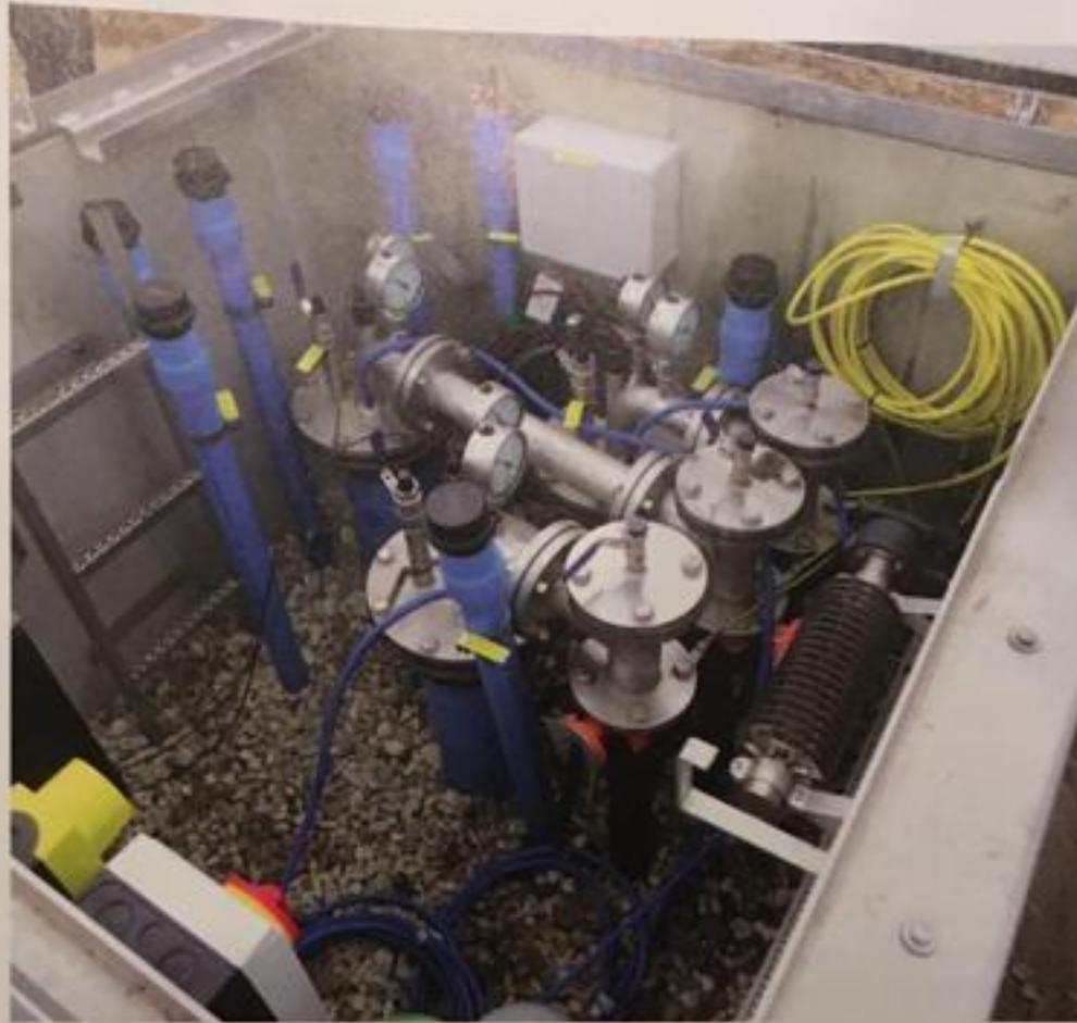
The main well has three screens that reach to the brackish zone at a depth of 90-110 metres under the dunes
